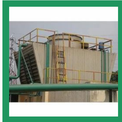
Timber Induced Draft Cooling Tower
