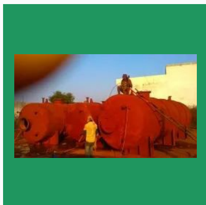
THERMAL STORAGE TANKS
